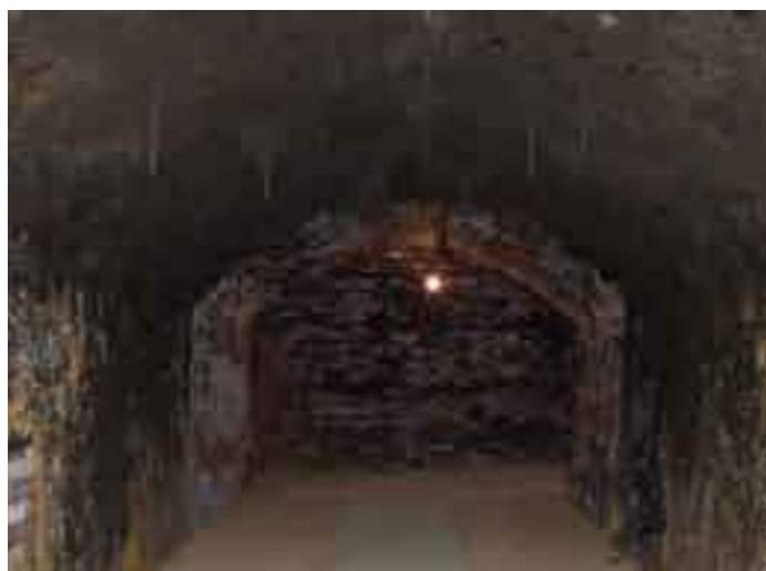
Fungus growing on the roof of one of the tunnels.
